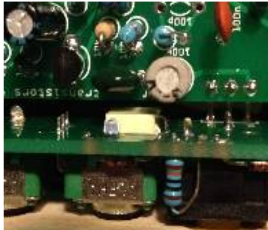
a 33n is bent flat against the board to make room for the electrolytic capacitor that looms over it
